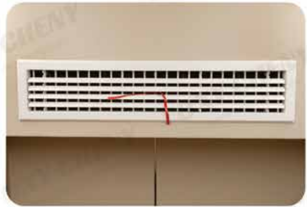
Air conditioner vent
