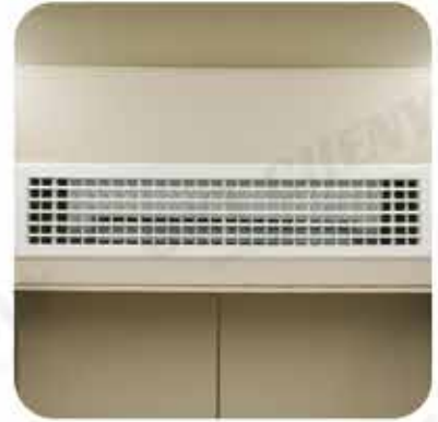
Air conditioner vent
